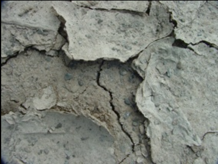
Desiccation cracks. Mould Bay.
