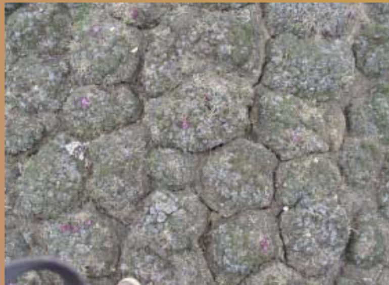
Contraction cracks, Green Cabin, Subzone C.
